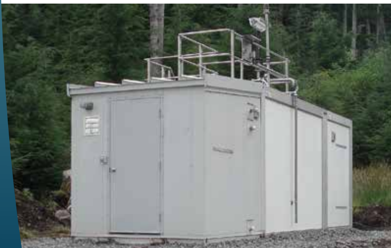
75 m 3 /day MBBR facility at the Queen Charlotte Lodge, BC.
